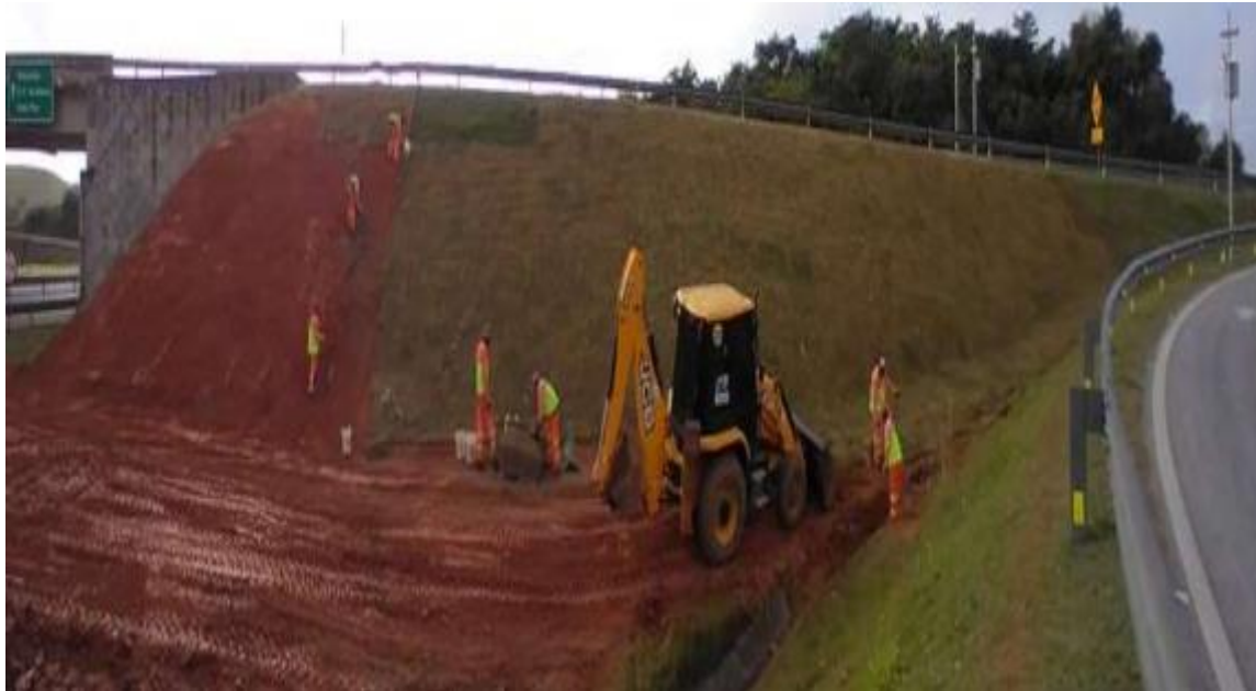
Figura 6.15 Via Lagos – Talude – Km 21+900 Norte
